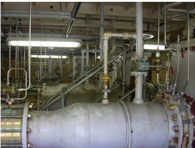
Pipework in the Building
